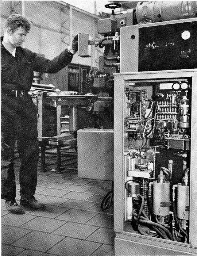
Fig. 4-19. (b) Close-up of welding equipment. Ignitrons are seen at bottom right and rotating wheel welding electrodes in front of the operator.
