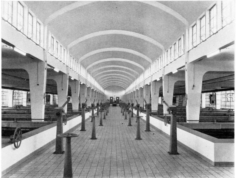
Fig. 4-43. General view of water purification room showing sand and gravel and flocculation filters.
