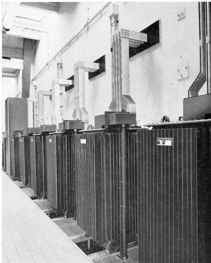
Fig. 4-56 (b) Three-phase power transformers.
