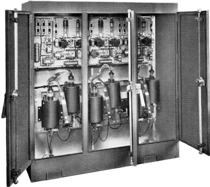
Fig. 4-39. (b) Main control cabinet housing ignitrons and ignition circuits.
